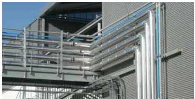
Outdoor installation Transair® 6" (168 mm)
